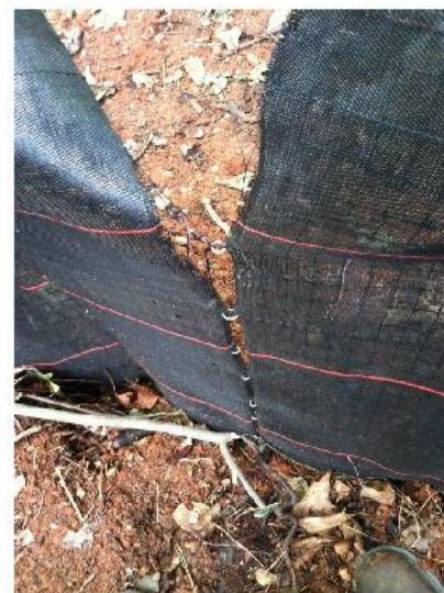
From factory, and installer didn't realize problem.
