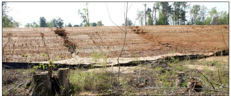
Failed slopes with no slope drains. Result, increase in workload and costs. Most importantly, offsite impacts and non-compliance issues can delay your project.
