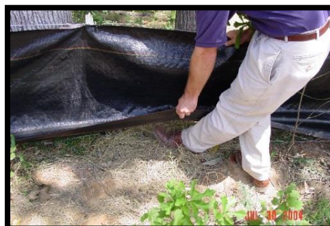
Failure to trench in silt fence
