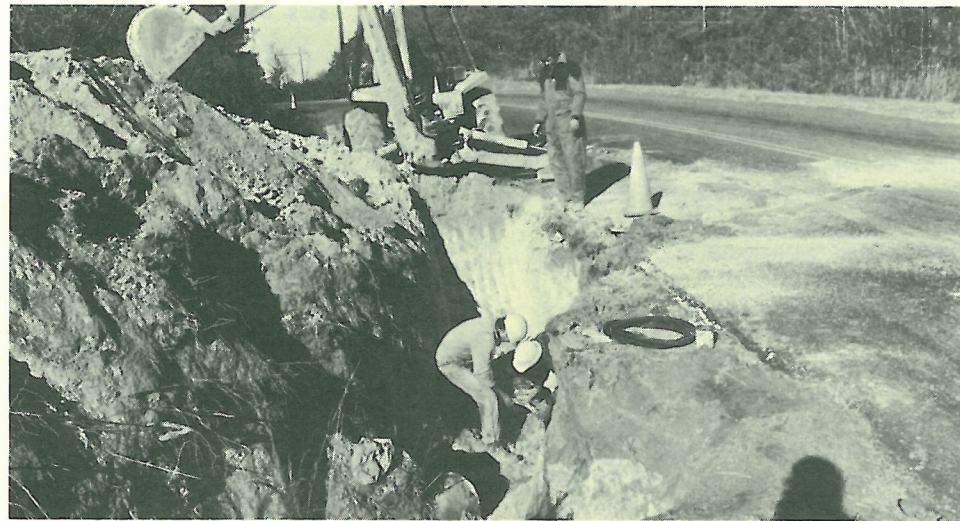
Water Line Improvements - Construction is nearing completion on the $475,000 Clay Street to Pisgah Road waterline and pump station project. When completed in early January, this project will more than double the City's upper level water system pumping capacity.
