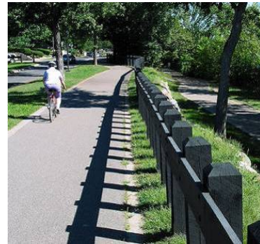
Wooden Safety Fence
