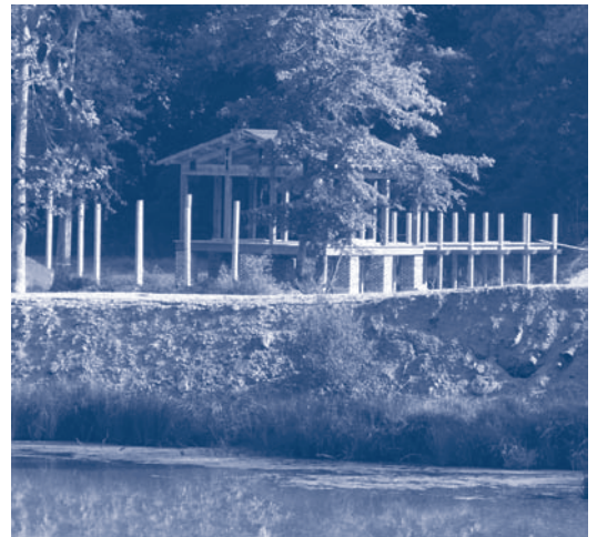
The completed pavilion (under construction in this photo) provides an opportunity to view the natural beauty of Brick Pond Park.
