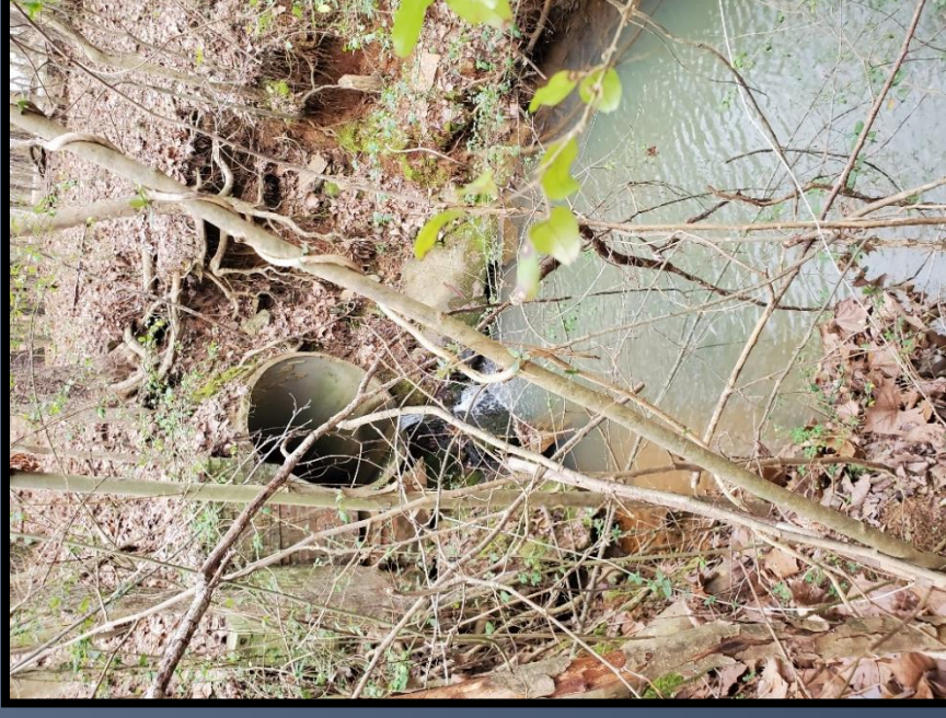
Downstream - below Bergen Road Failing infrastructure
