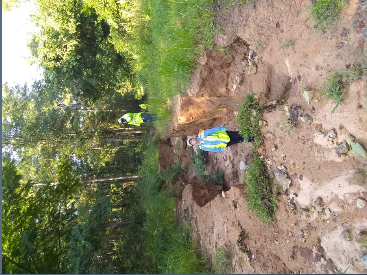
After storm blows out repairs – August 2021
