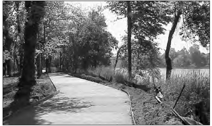
Construction is nearing completion on the Riverfront Greenway extension. Users will enjoy close proximity to the Savannah River, seen here to the right of the trail.
