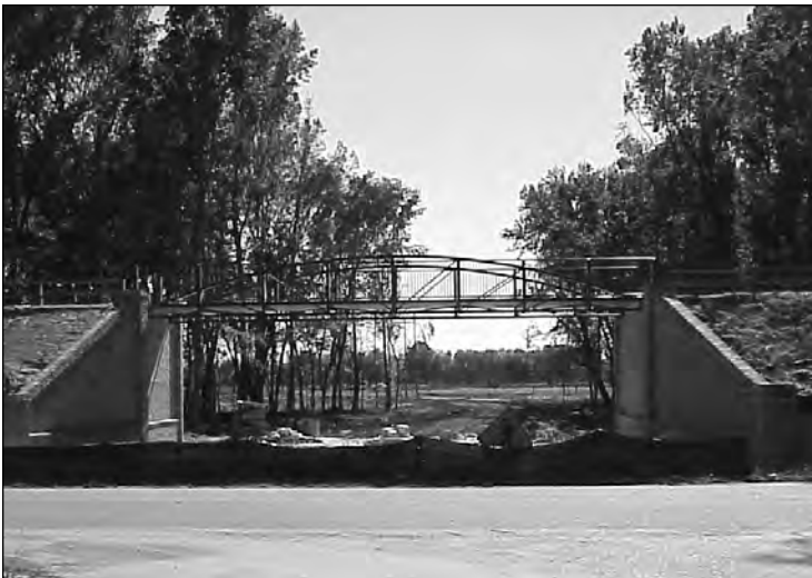
The new Greenway pedestrian bridge crosses the Crystal Lake Drive extension into the Hammond's Ferry development. The installation of storm drains along the roadway extension is currently underway.
