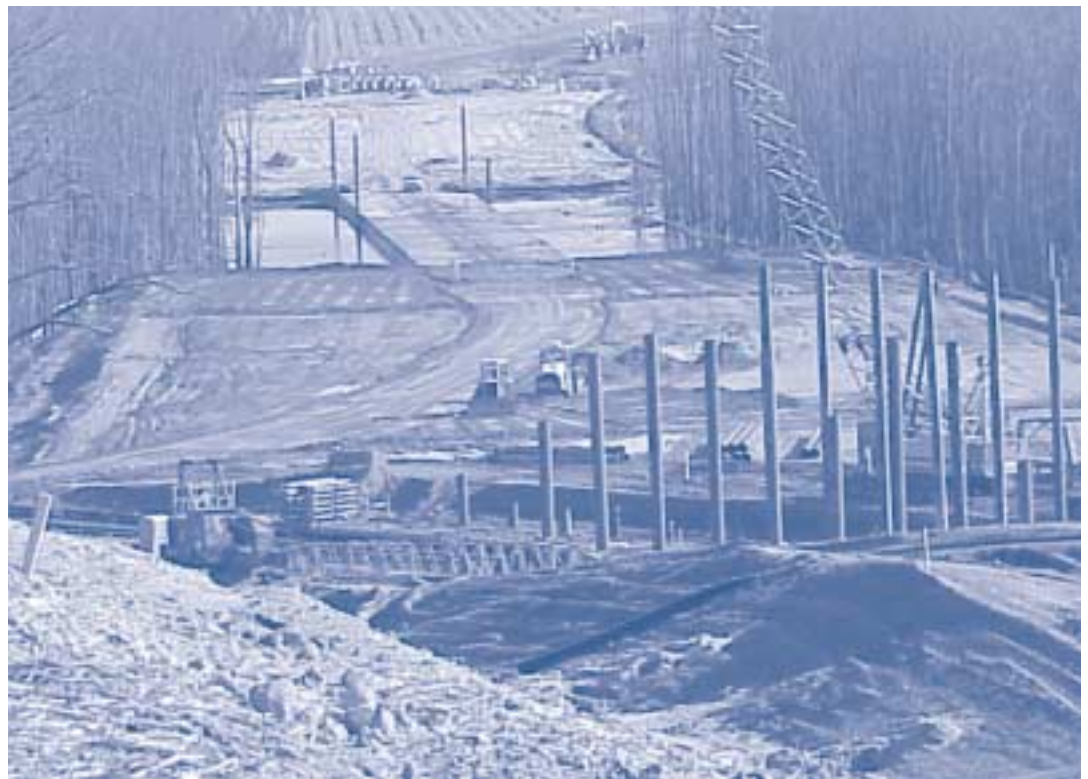
Last month the South Carolina General Assembly passed a local bill that officially changes the name of I-520 on the South Carolina side of the Savannah River, shown here under construction, from Bobby Jones Expressway to Palmetto Parkway.
