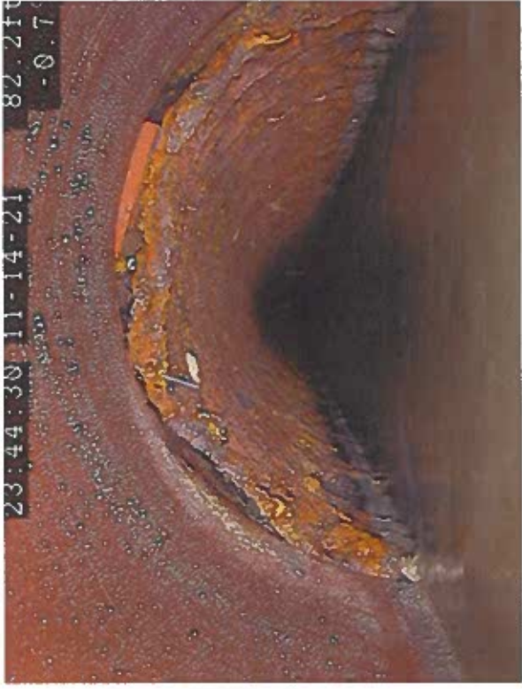
Before - 18" Corrugated Metal
