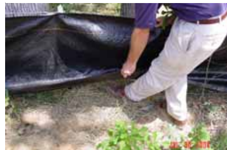
FIGURE E-22 SILT FENCE FAILURE
