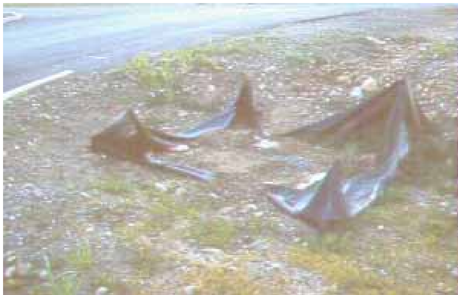
IMPROPERLY INSTALLED AND UNMAINTAINED SILT FENCE DROP INLET BARRIER
